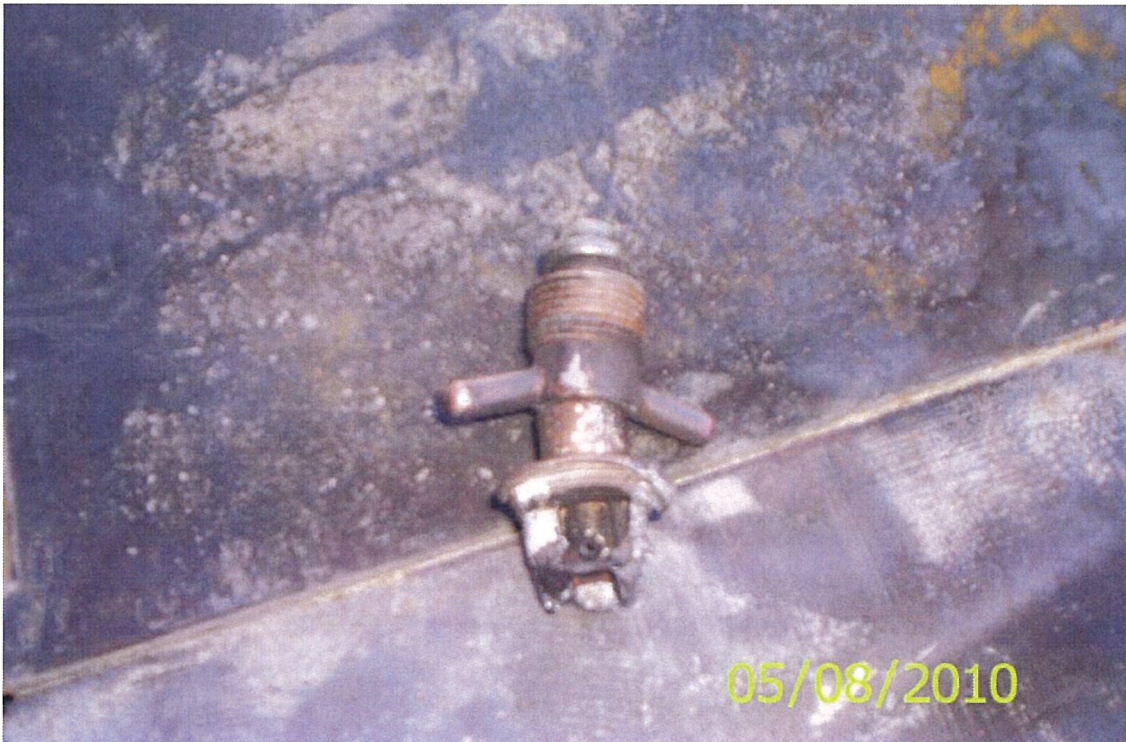
Fire damage to the gas fitting for LPG Cabinet Heater
