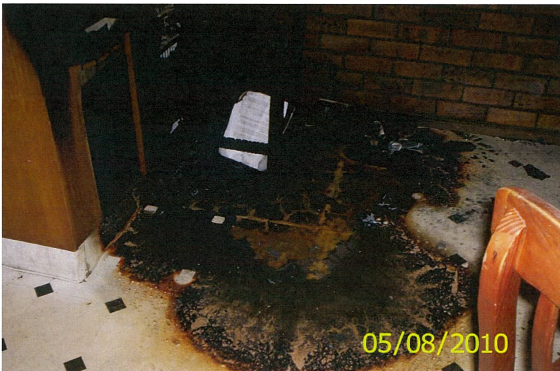
Fire damage in kitchen/dining area due to LPG Cabinet Heater
